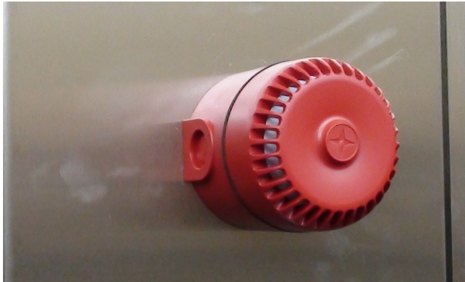
Figure 264: Safety horn on the machine paneling
