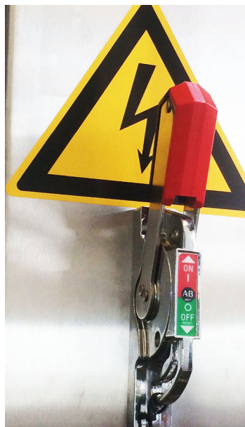
Figure 198: Main switch for the power supply on the switch cabinet
